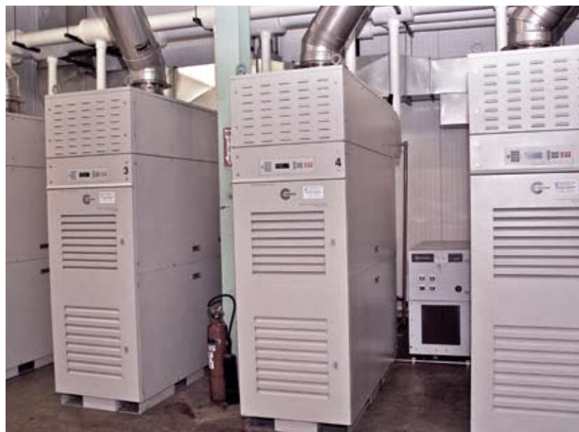
Capstone microturbines provide cooling, heating and power at Astor Chocolate in New Jersey.
